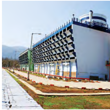
Induced draft cooling tower, Kaiga
