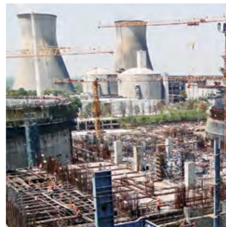
Kakrapar nuclear power plant
