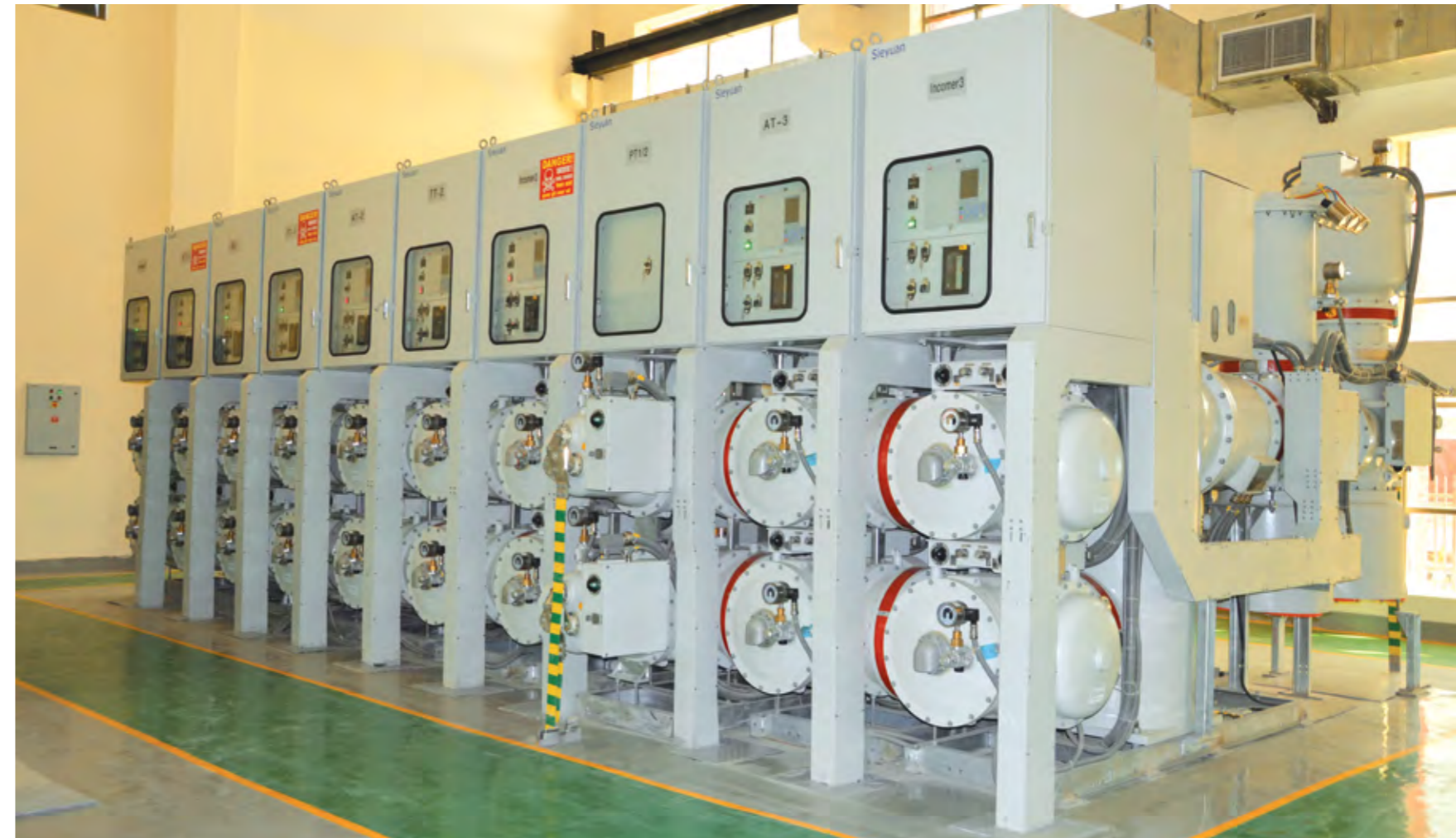
Receiving substation powering Lucknow Metro
