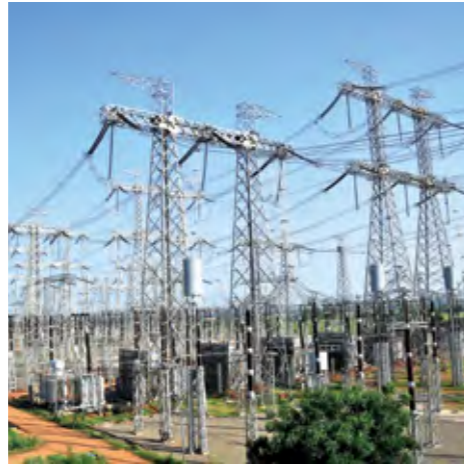
765 kV ultra high voltage AIS at Unnao
