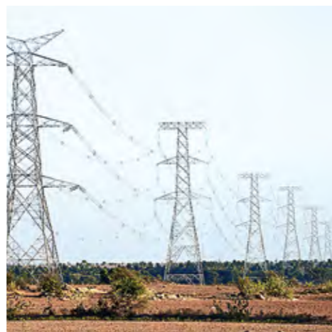
765 kV D/C transmission line at Kudgi
