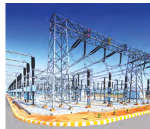
220 kV switchyard at Ranchi for PGCIL
