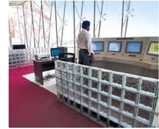
Inside view of the control room
