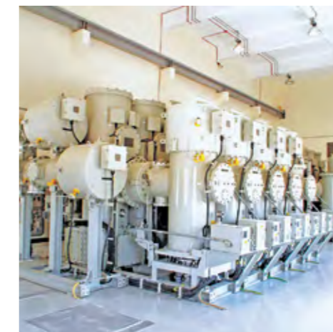
132 kV GIS for Salah power plant, Oman
