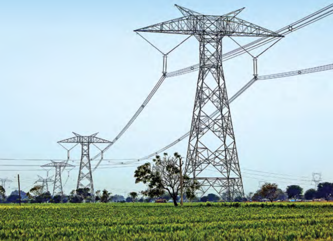
800 kV HVDC Nidhura - Agra transmission line
