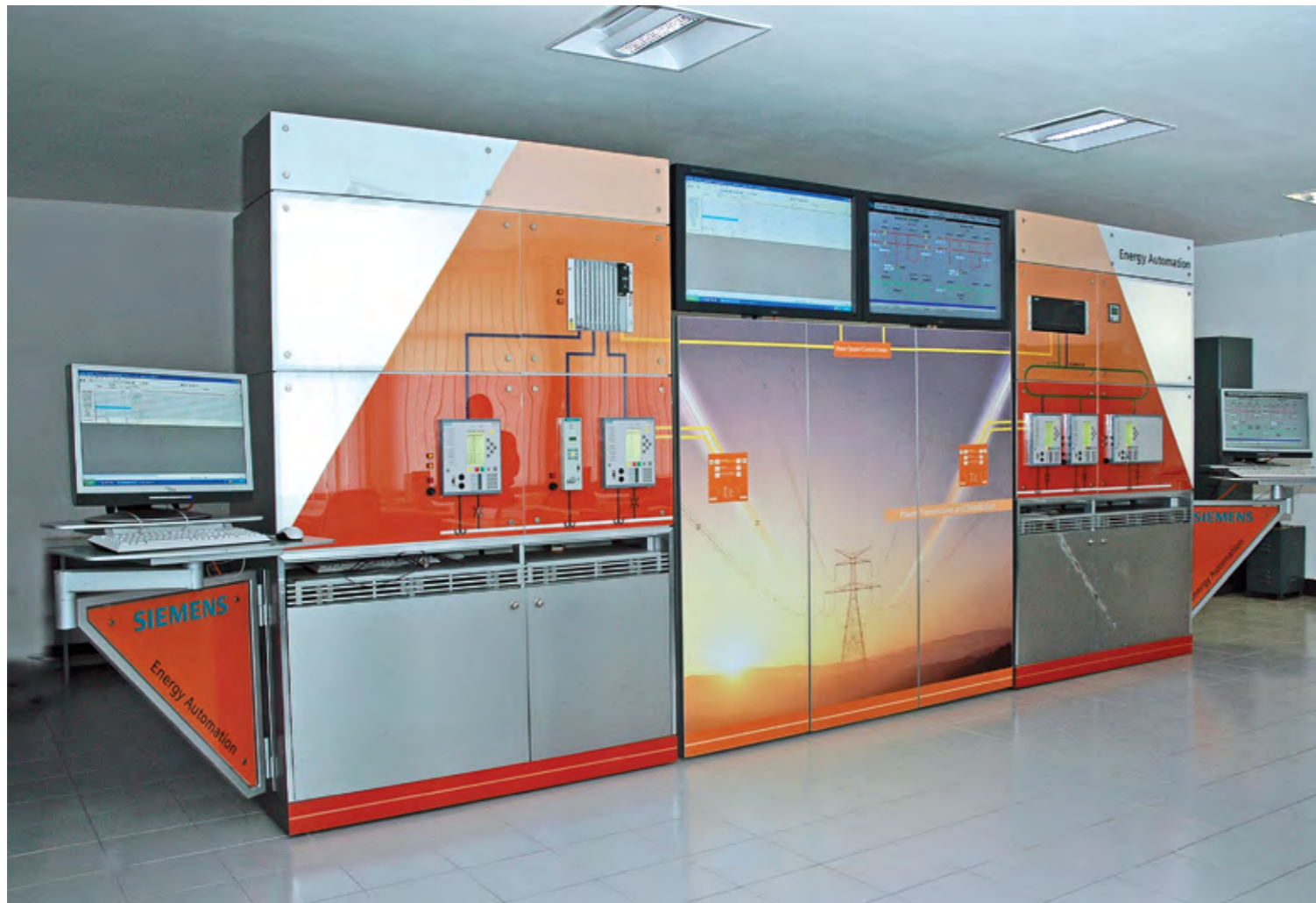
Substation Automation System display panel at L&T's training lab in Chennai
