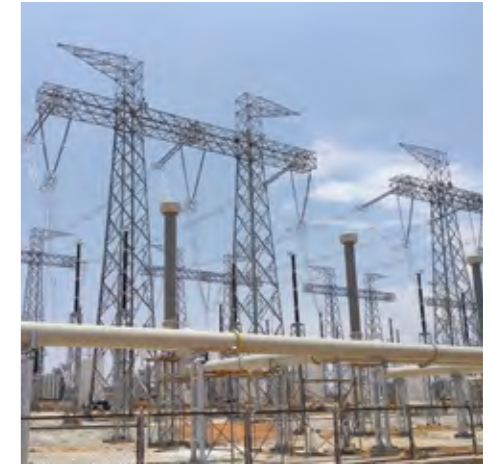
765 kV GIS, Hyderabad
