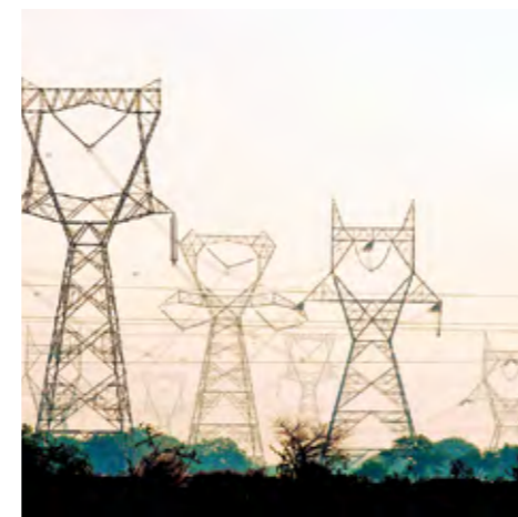
765 kV Sipat - Seoni transmission line
