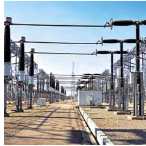
400 kV switchyard for Jindal Power Plant
