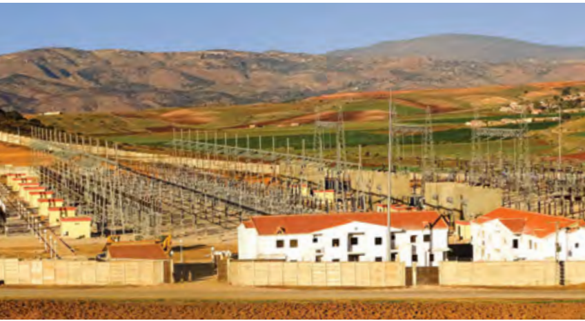
400 kV AIS at Chlef in Algeria
