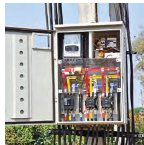
Rural Load Management System (RLMS)
