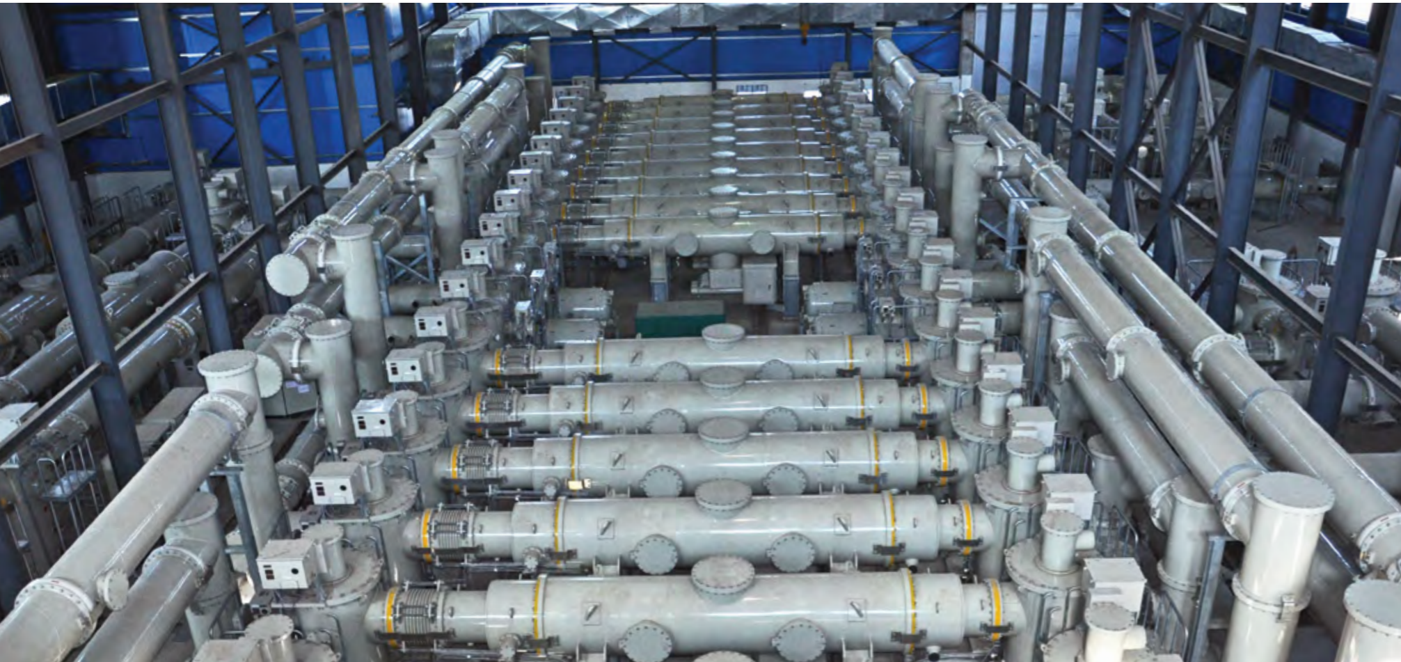
765 kV GIS at Pune
