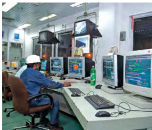
Control system for a sinter plant
