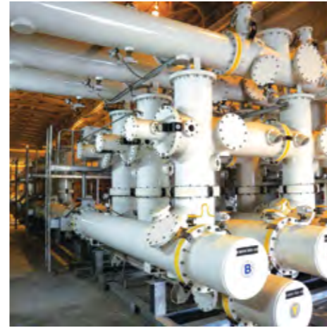
400 kV GIS switchyard at Chennai
