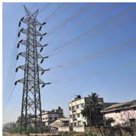
Multi-circuit narrow base transmission line tower for Mumbai
