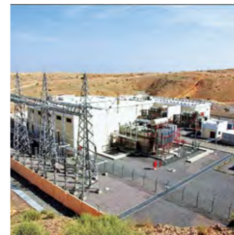
220 kV grid substation at Airport Heights, Oman
