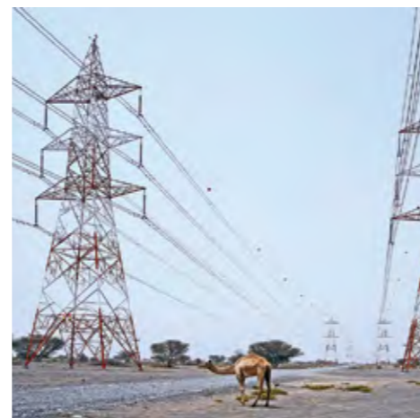
220kV transmission line for Blue City project at Muscat, Oman
