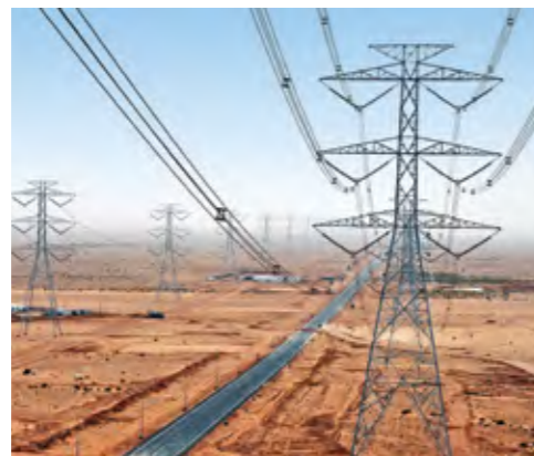
380 kV transmission line at Riyadh in Saudi Arabia
