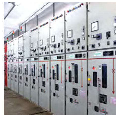
Switchgear panels for a steel plant
