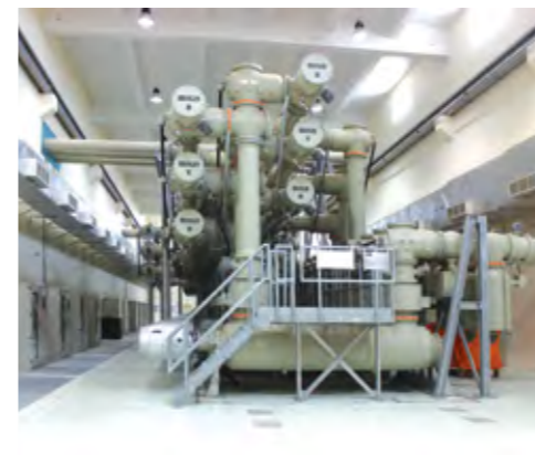
400/220/132 kV substation at Izki in Oman
