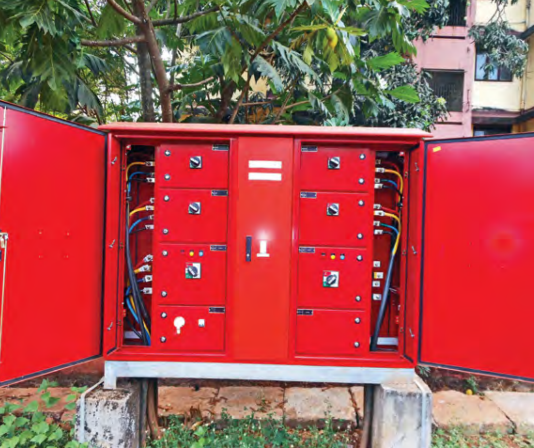
Power control panels
