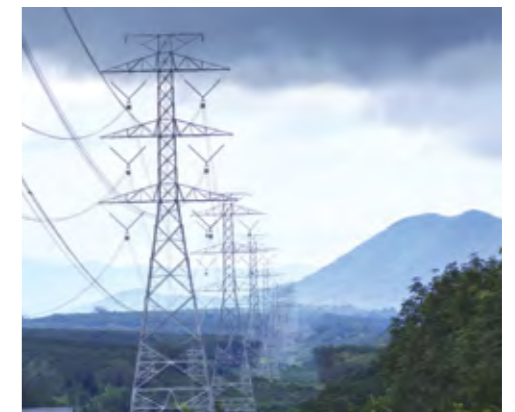
500 kV Tha Li-Khon Kaen 4 transmission line, Thailand
