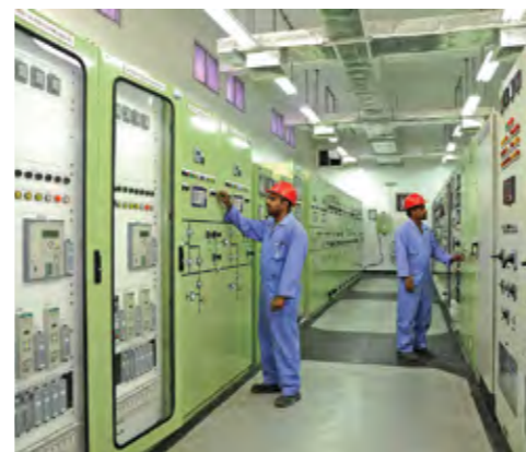
Control panels at a substation
