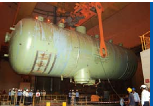
2 x 1000 MWe Kudankulam Nuclear Power Plant
