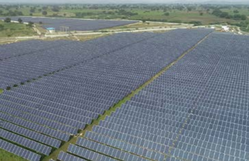
209 MWp/190 MW Solar Tracker Project, Karnataka
