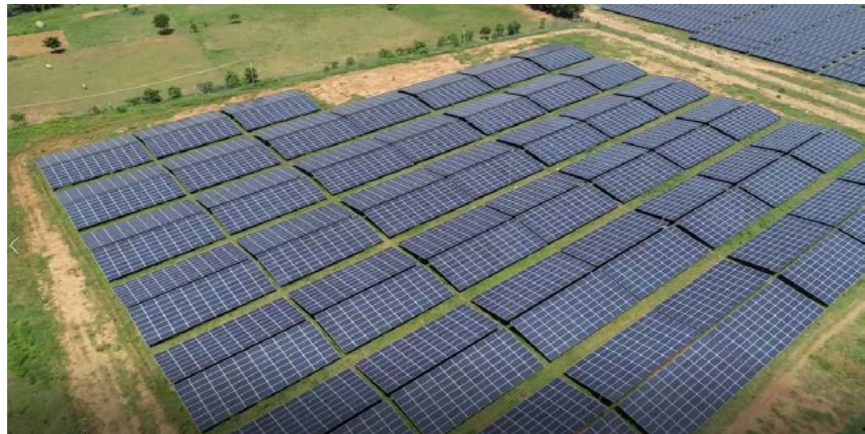
2.5 MWp East-West Solar PV Plant
