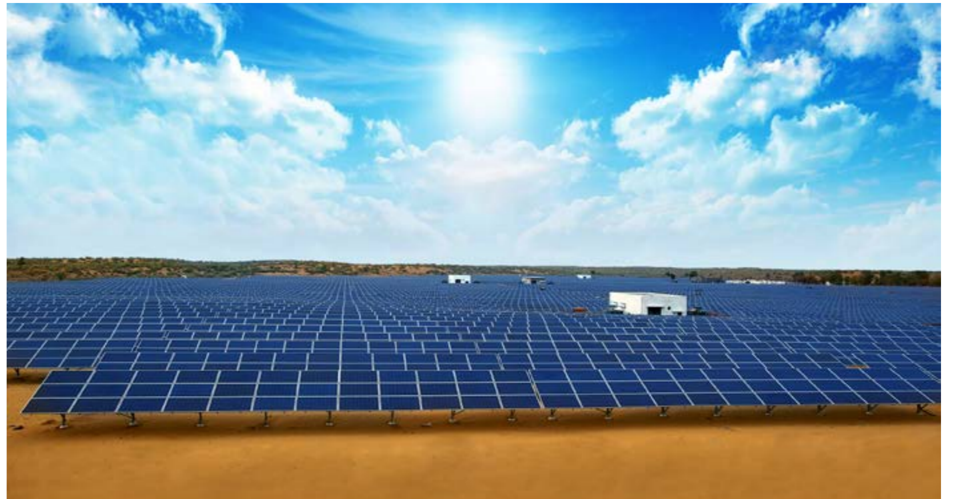
22 MWp Solar PV power plant at Rajasthan
