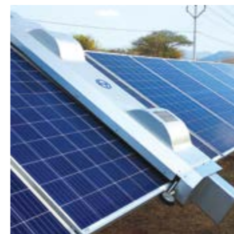
Automatic dry cleaning of solar PV modules
