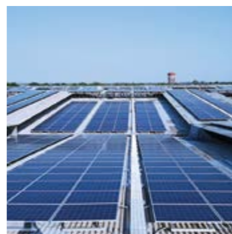
7.5 MWp solar rooftop PV system at Beas, Punjab
