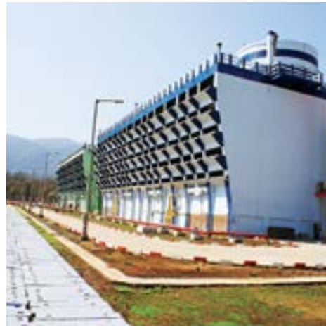
Induced draft cooling tower, Kaiga
