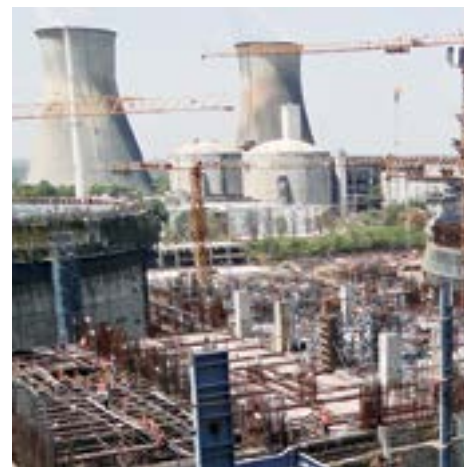
Kakrapar nuclear power plant
