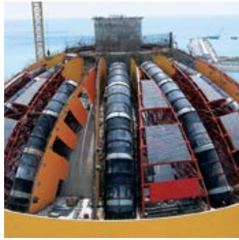
Kudankulam nuclear power plant
