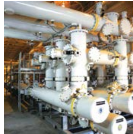
400 kV GIS switchyard at Chennai
