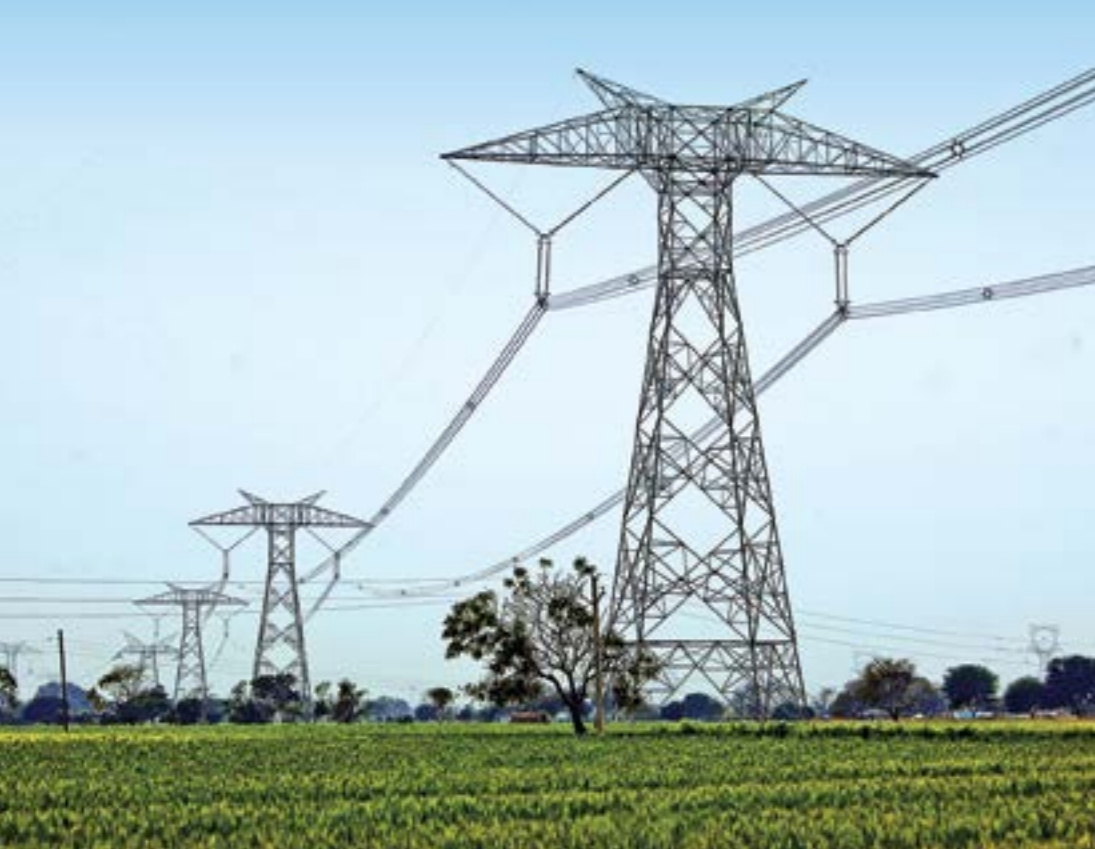
800 kV HVDC Nidhura - Agra transmission line
