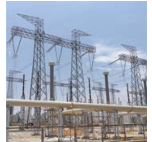
765 kV GIS, Hyderabad
