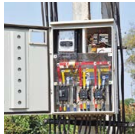
Rural Load Management System (RLMS)
