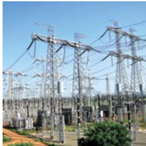
765 kV ultra high voltage AIS at Unnao
