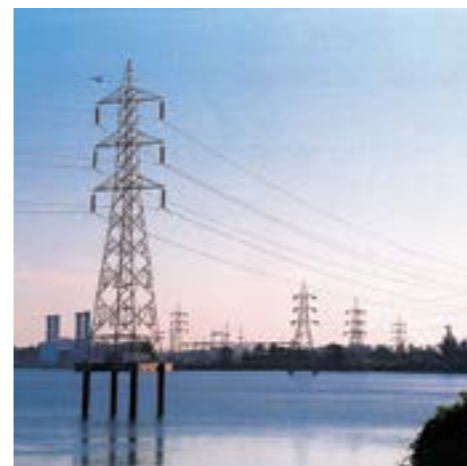
220 kV river crossing transmission line on pile foundations
