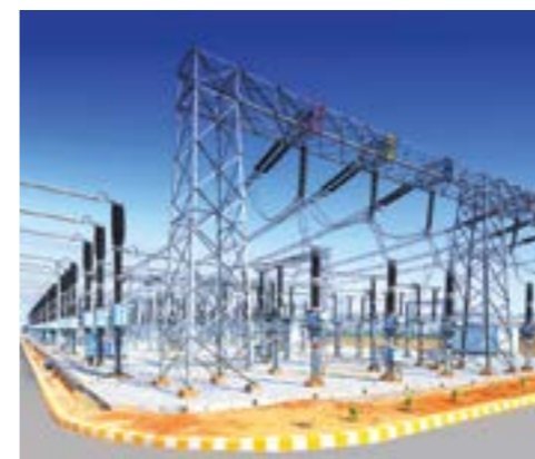
220 kV switchyard at Ranchi for PGCIL
