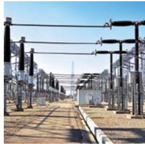
400 kV switchyard for Jindal Power Plant
