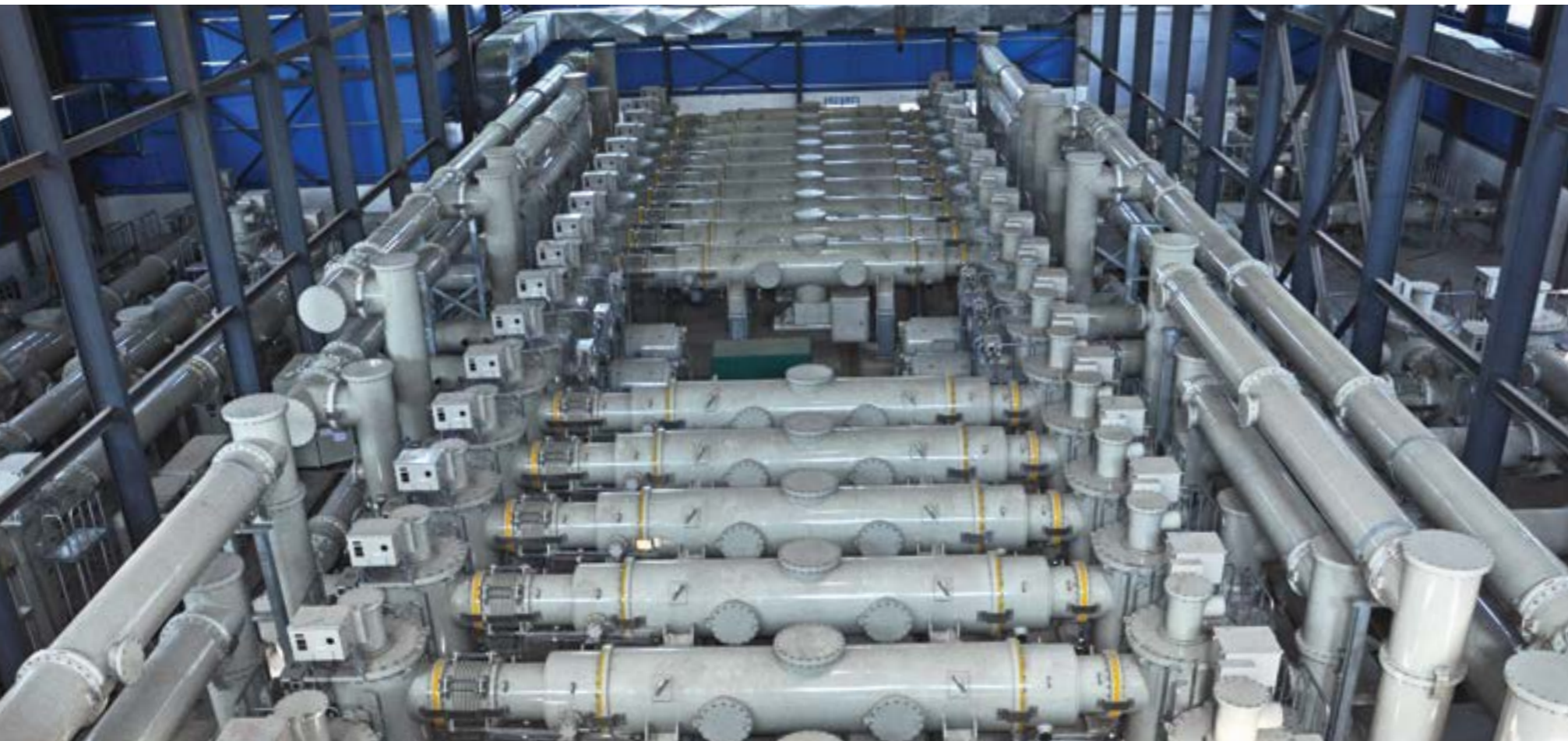
765 kV GIS at Pune
