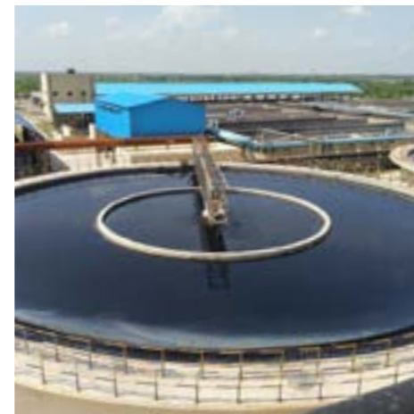
100 MLD Common Effluent Treatment Plant, Narol, Gujarat
