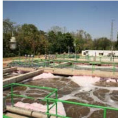
Wastewater Treatment Plant at the President's Estate, New Delhi
