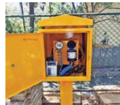
District meter cabinet
