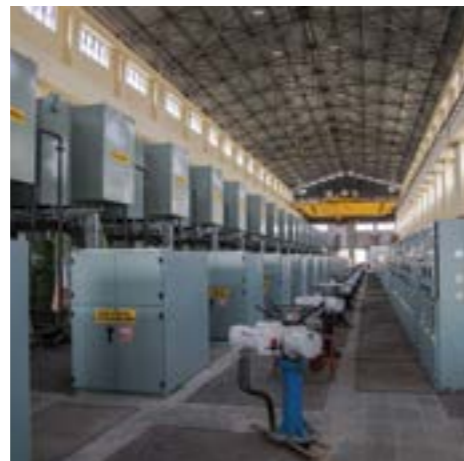
Pump house at Hanamapur, Karnataka
