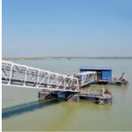
Floating barge intake, Sahibganj, Jharkhand
