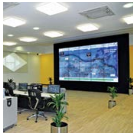
Real-time Project monitoring with SCADA
