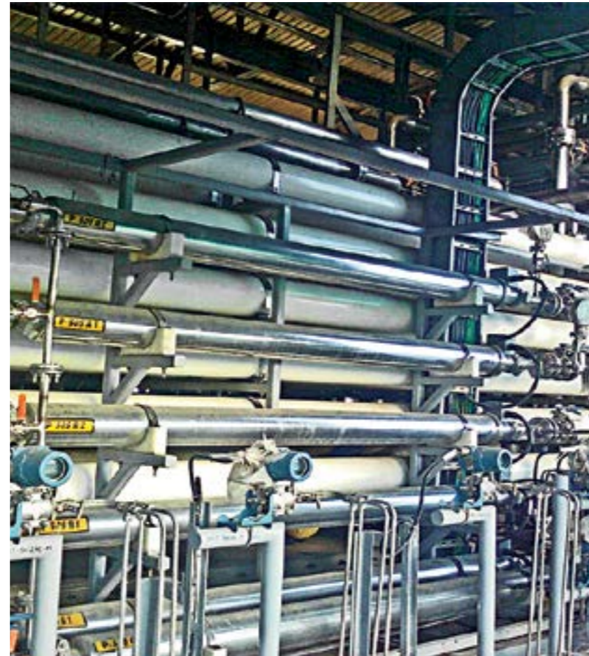
Reverse osmosis technology at a desalination project
