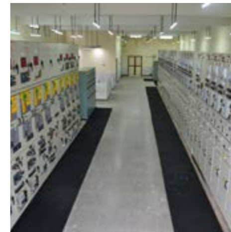
Substation, Bidkin, Maharashtra
