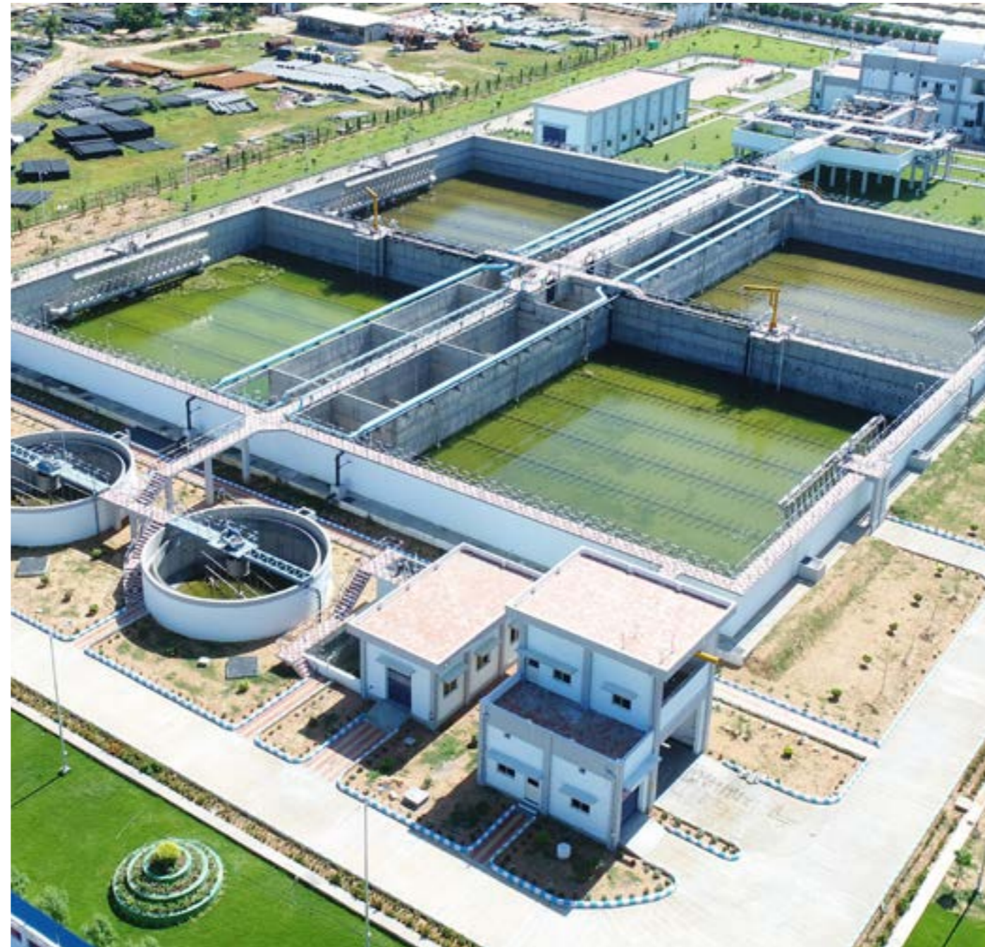
55 MLD Wastewater Treatment Plant, Nellore, Andhra Pradesh
