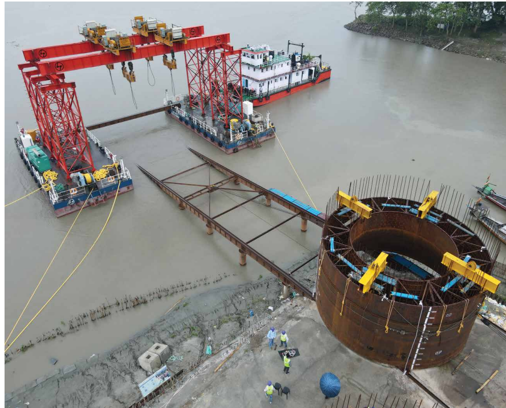
Launching a caisson (right) in the Brahmaputra to bore wells for erecting bridge piers.
