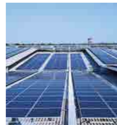
7.5 MWp Solar Rooftop PV System at Beas, Punjab
