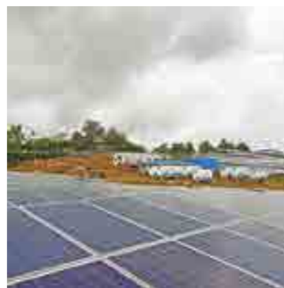
2x11 MWp with 16 MW/8MWh Battery Energy Storage System, Andaman
