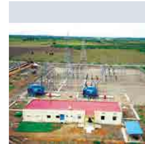
HV Substation and Transmission
