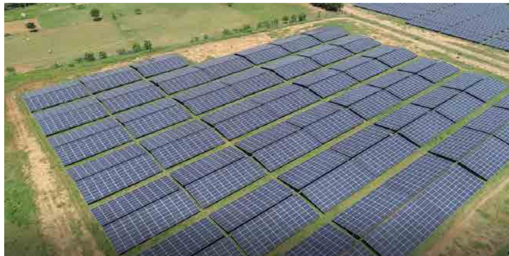
2.5 MWp East-West Solar PV Plant
