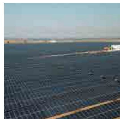
324 MWp Fixed Tilt Solar PV Project at Rewa Ultra Mega Solar Park (RUMS), Madhya Pradesh
