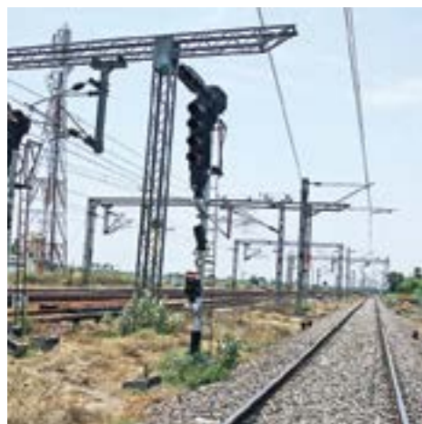
Signaling and telecommunication
