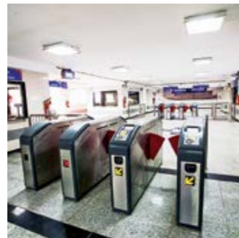
Automatic ticketing system at Mumbai Monorail
