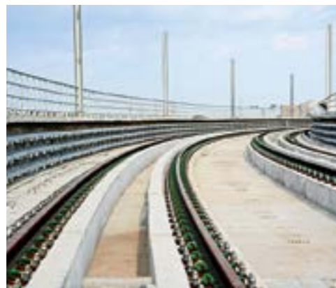
Ballastless track at Chennai Metro
