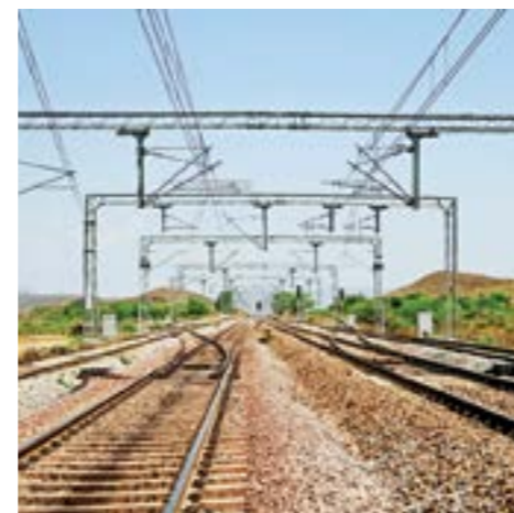
Railway sidings for Dhamra port
