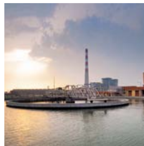
Plant Water System, Sagardighi, West Bengal
