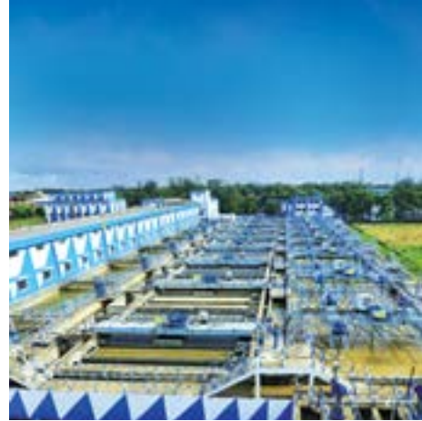
227 MLD Water Treatment Plant at Garden Reach, Kolkata, West Bengal
