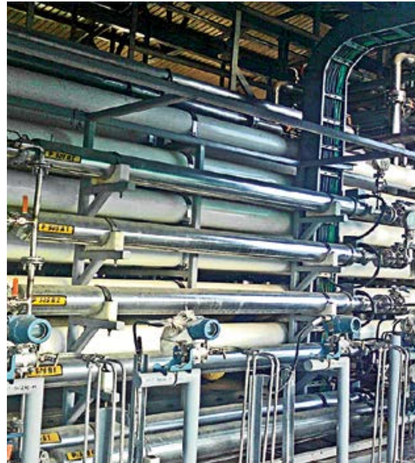
Reverse osmosis technology at a desalination project
