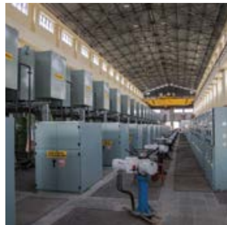
Pump house at Hanamapur, Karnataka
