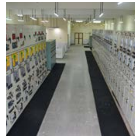
Substation, Bidkin, Maharashtra
