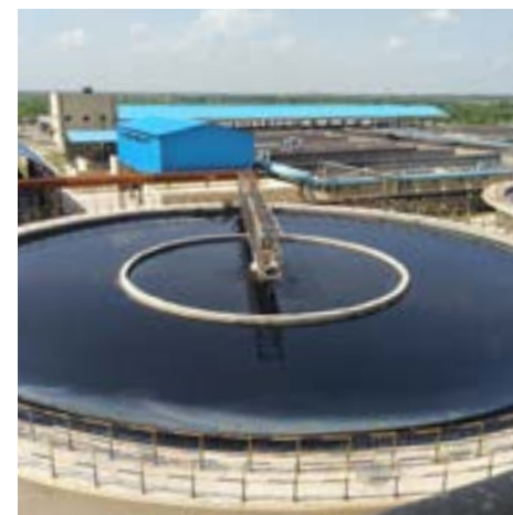
100 MLD Common Effluent Treatment Plant, Narol, Gujarat
