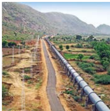
Transmission Mains, Bisalpur, Rajasthan
