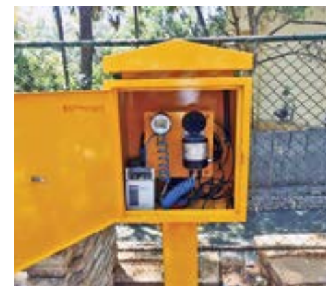
District meter cabinet
