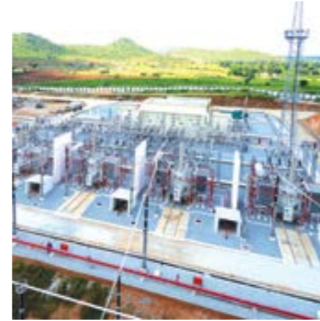
India's first STATCOM at NP, Kunta, Andhra Pradesh
