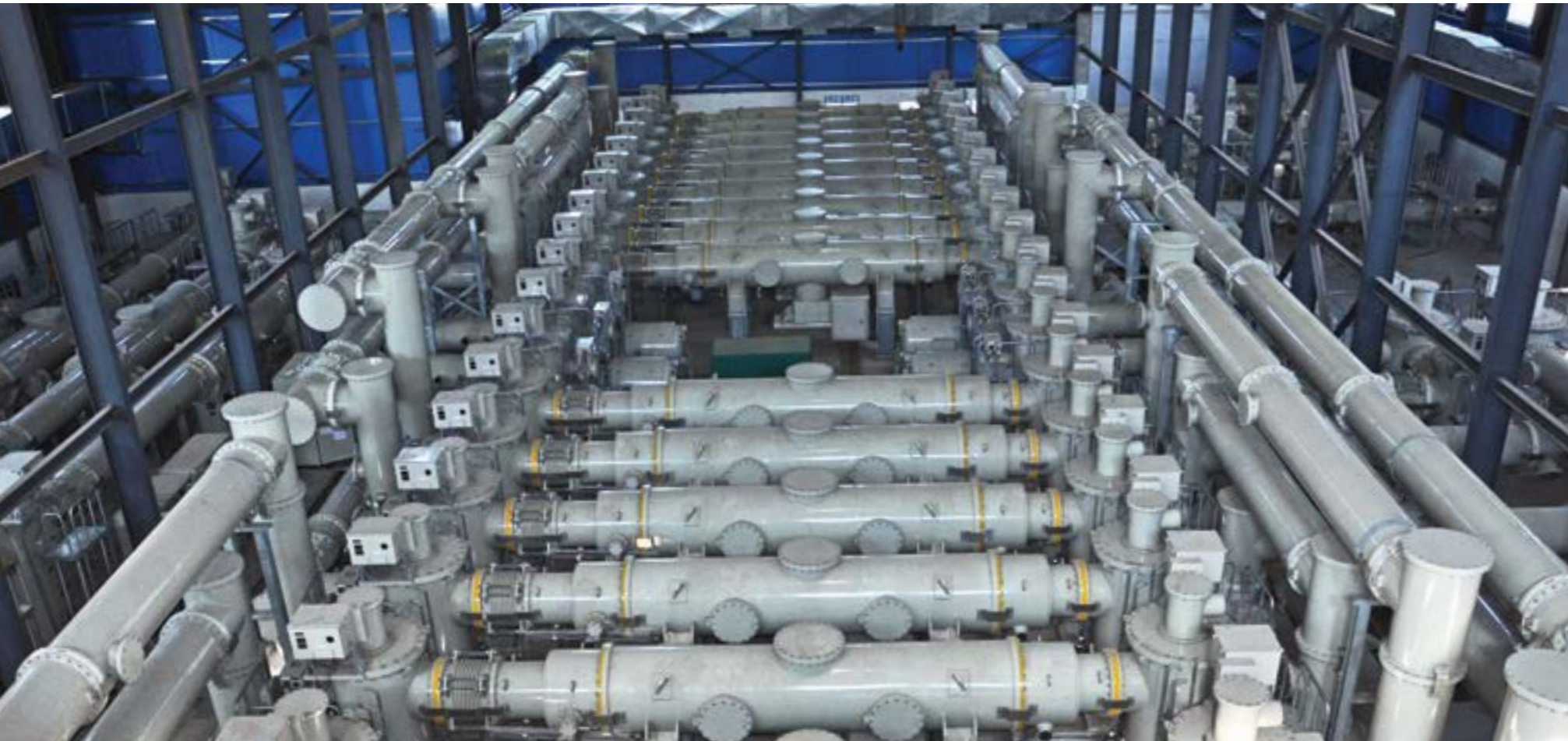
765 kV GIS at Pune
