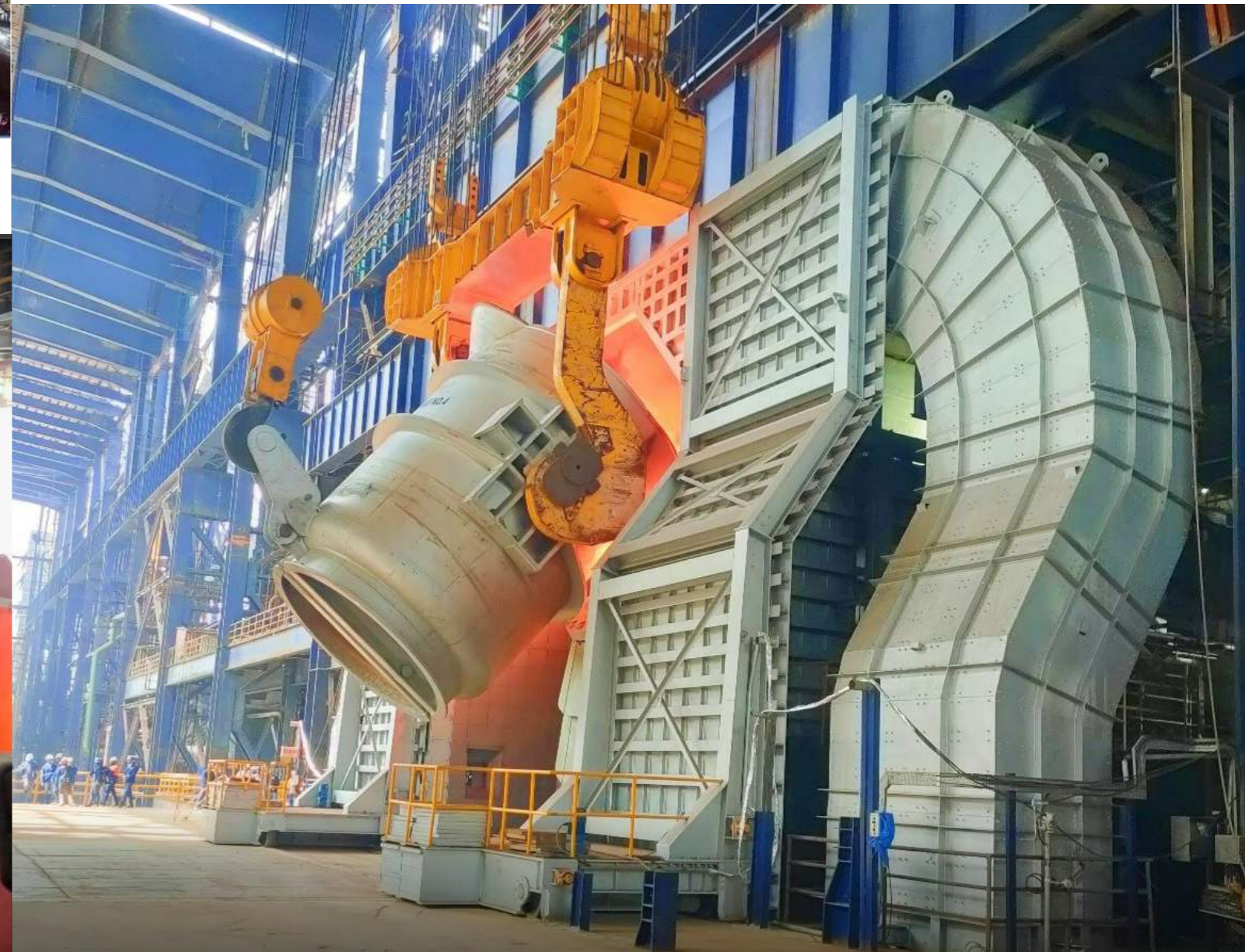
Steel Melt Shop #2 – 350 t Converter 1 at JSW Dolvi
